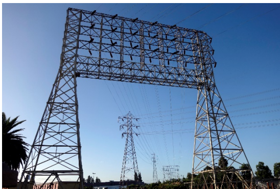
Figure 3: High-voltage distribution will have capacity for EV charging.
